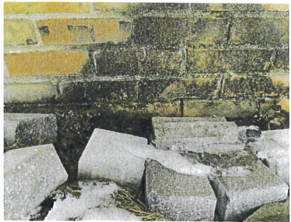
Photo 7: Block erosion below NW roof drain
