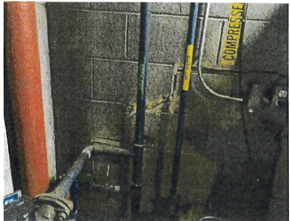
Photo 8: SW interior wall local settlement
