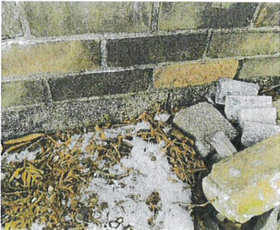
Photo 6: Block erosion below SW drain
